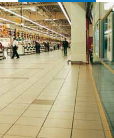
An example of an installation with Keraquick in an Auchan supermarket - Sosnowiec (Poland)
